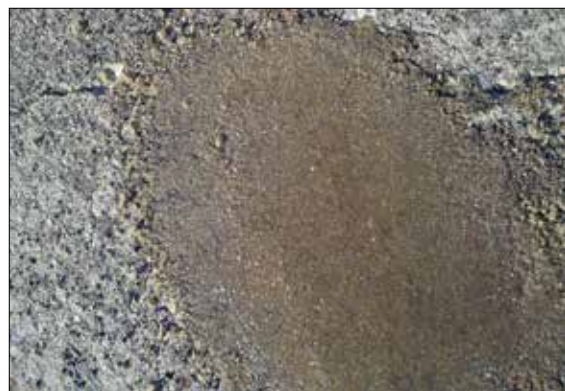
Pit patched with epoxy and sand
