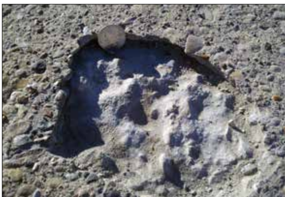
Pit in concrete
